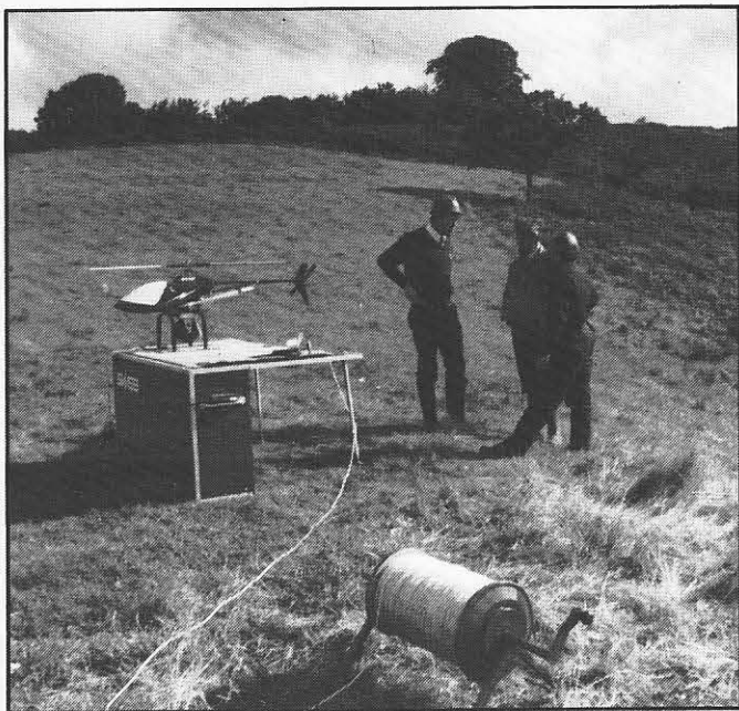
This is how it's done. Here we can see the model on its integrated carrying case and heli-pad. In the foreground is the reel which is carrying the heavy line which will be used to, eventually, pull across the power line.
